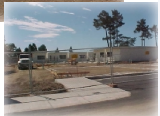
Demolition of old structures, grading the site and the new, permanent portable buildings for Ark High Students
